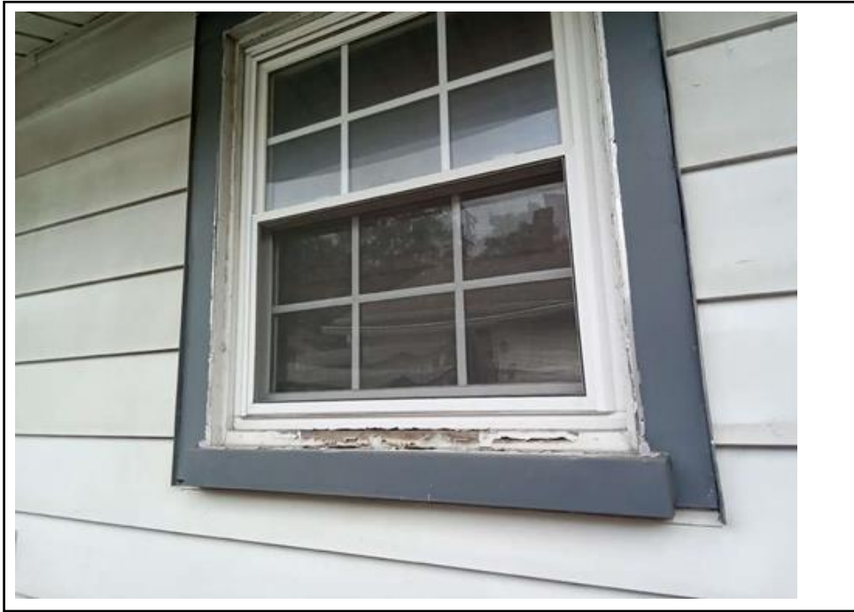
peeling paint on trim
