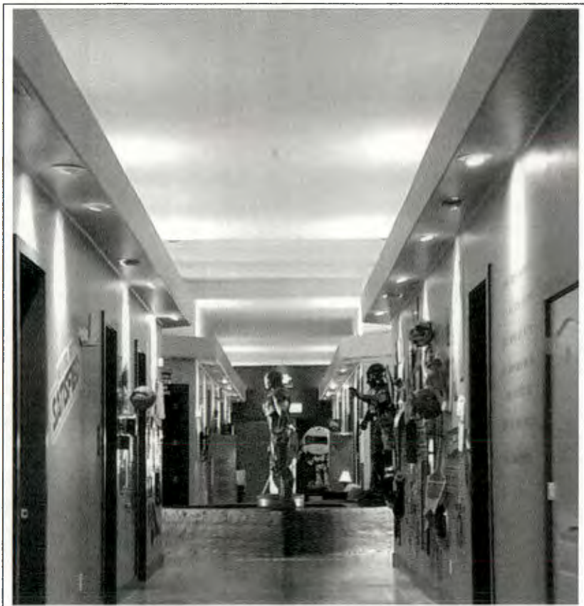
Before – Hallway blocked with large Star War figures and phone booths – Safety Hazard-
